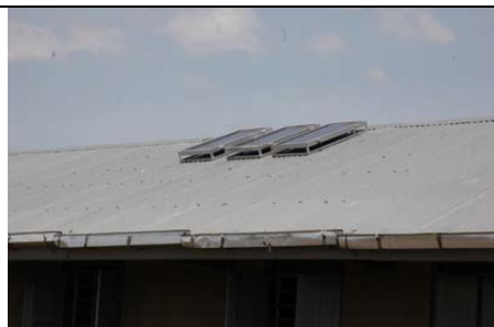
Three solar panels on the school roof
